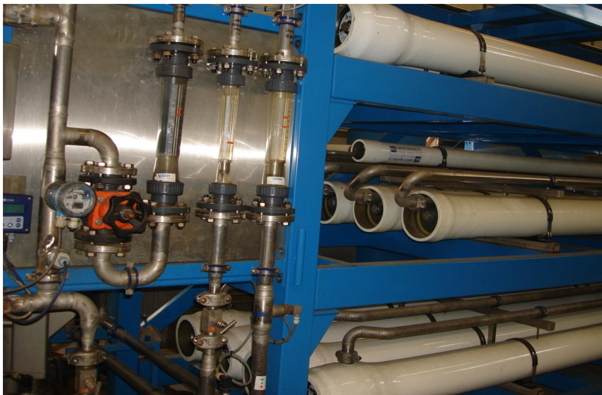
Picture C.9: Reverse osmosis unit.
