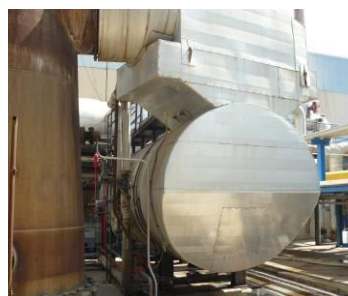
Picture E.9: Boiler (heat recovery)
