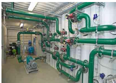
Picture A.6: Valve pit.
