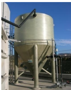
Picture D.7: Settling separator
