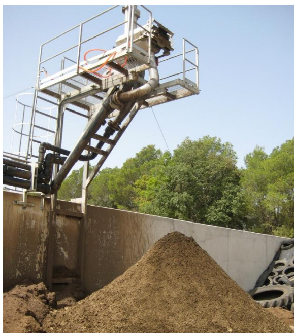
Picture G.5: Mechanical separator
