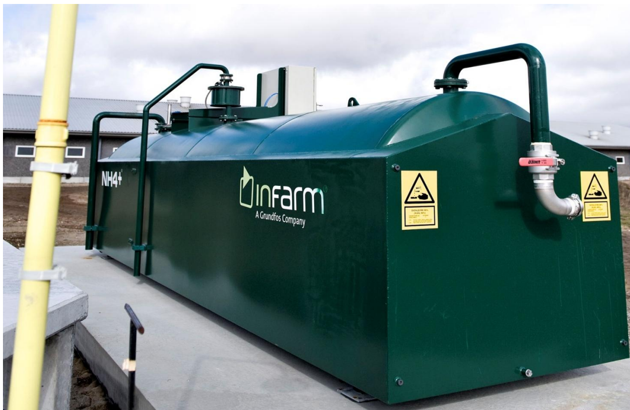
Picture B.1: Acid tank
