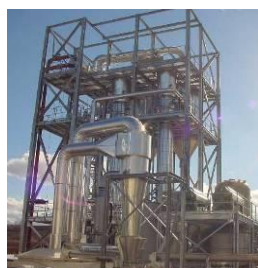
Picture E.5: Vacuum evaporation towers
