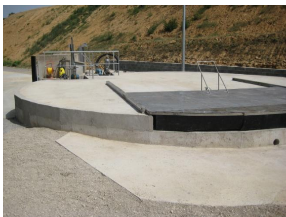
Picture G.3: Reception tank of slurry
