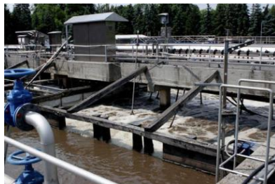
Picture F.8: WWTP Domžale-Kamnik
