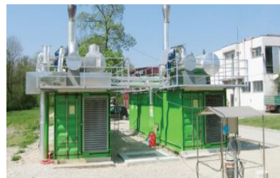
Picture F.6: CHP engines
