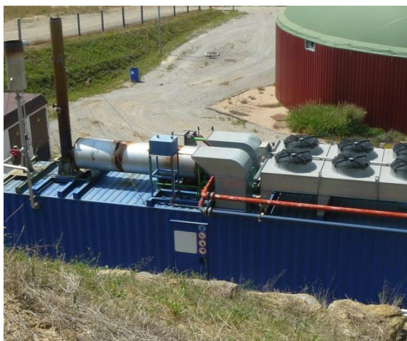
Picture G.7: Container with CHP engine
