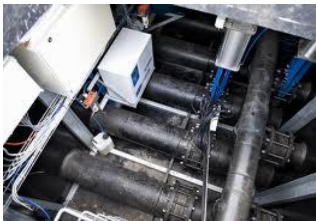
Picture B.2: Valve pit
