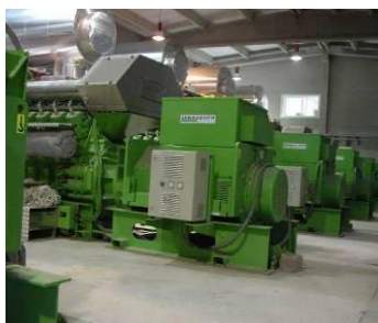
Picture E.8: CHP engines
