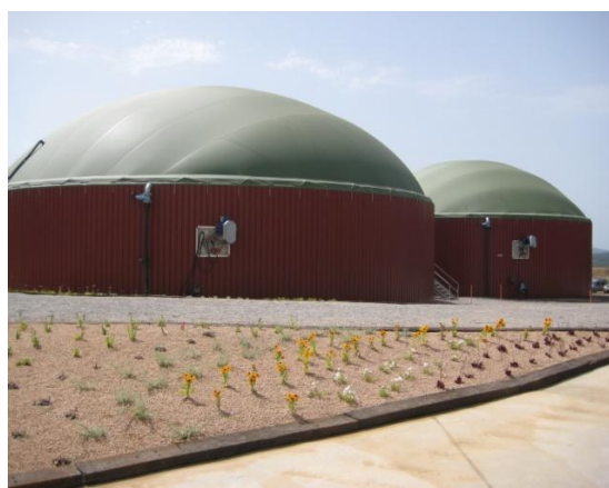
Picture G.4: Anarobic digesters
