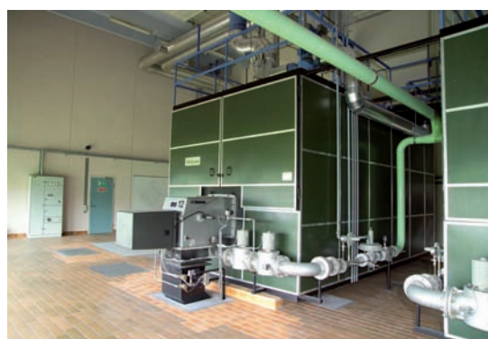
Photo: Hollensen Energy
