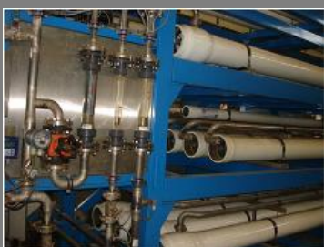
Installation for reverse osmosis of liquid separation fractions.
